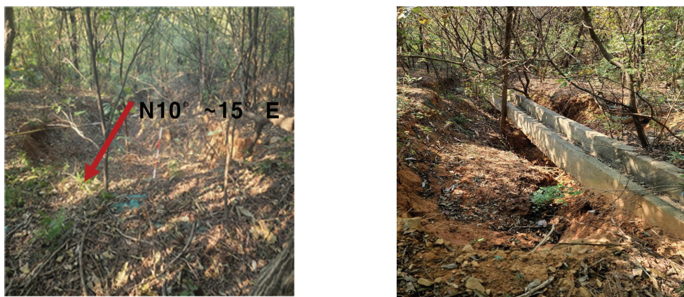
Figure 3. The actual condition of slopes of hillsides that have collapsed due to land creep.
