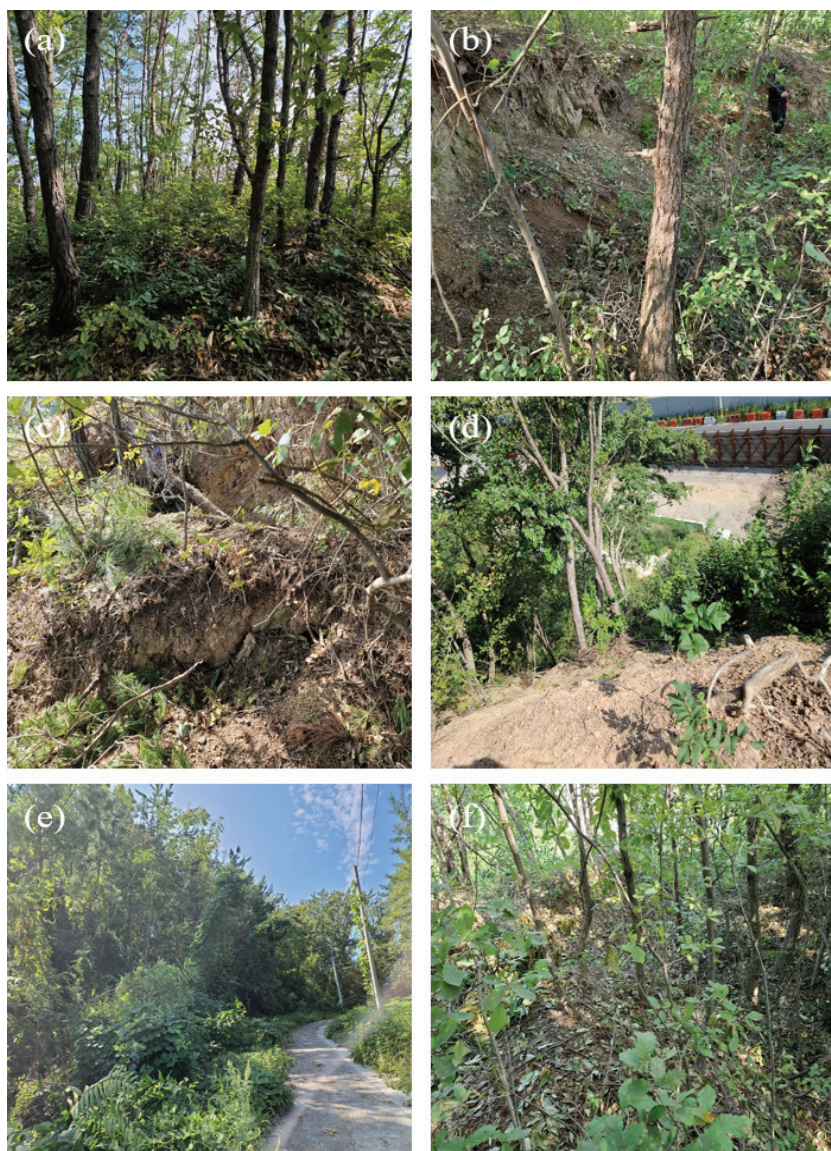
Figure 7. a, concave type of the top part; b and c, tensile crack; d, concave type of groundwater inflow point; e, soil displacement caused by landcreep; f, water catchment in the lower road.
